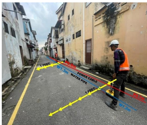
Tracing officers identifying the number of utilities present underground using induction method of PCL
