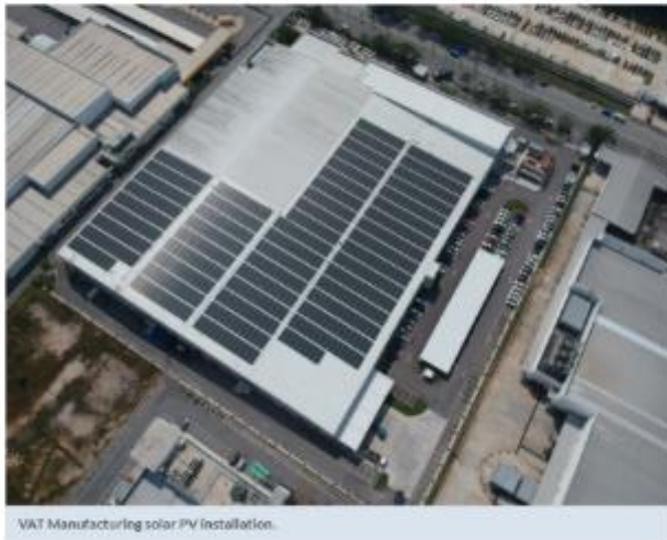
VAT Manufacturing solar PV installation.
