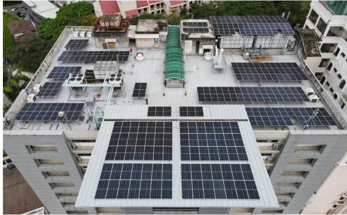
Donated a 154.4kWp solar PV system to Tung Shin Hospital with O&M
