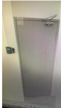
FIRE-RATED DOOR FOR STAFF SAFETY
